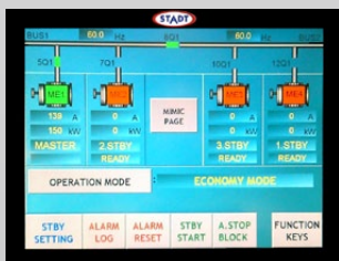
Power Management System
