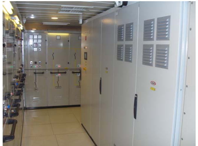
ALSO FROM MAIN SWITCHBOARD ROOM
