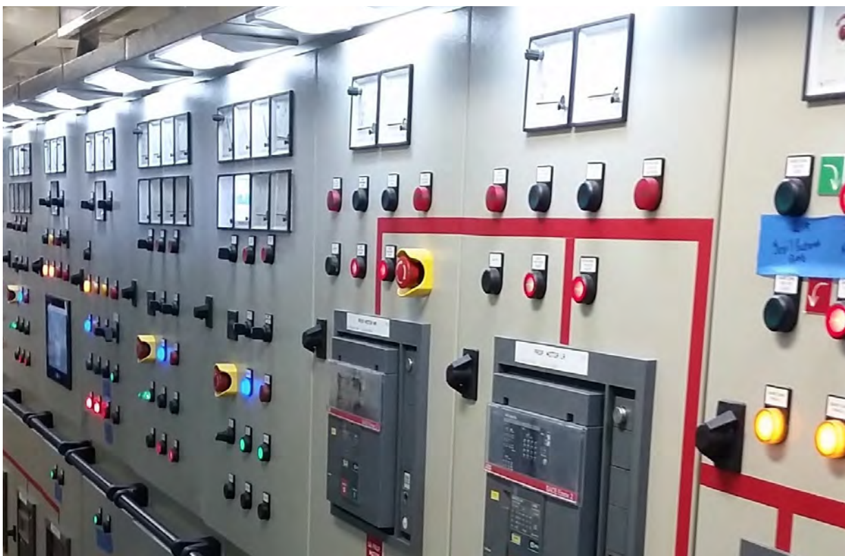
STADT Main Switchboard
