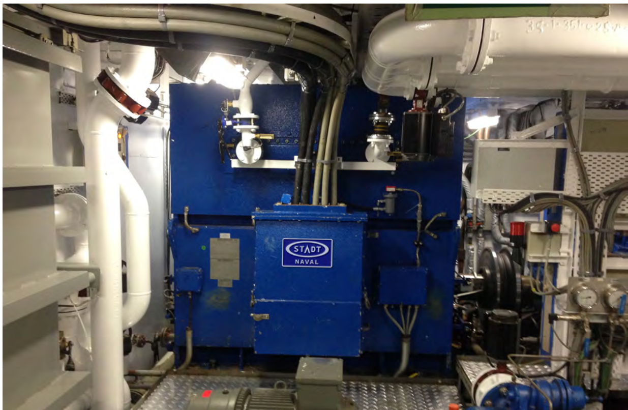
Main Propulsion Electric Motors
